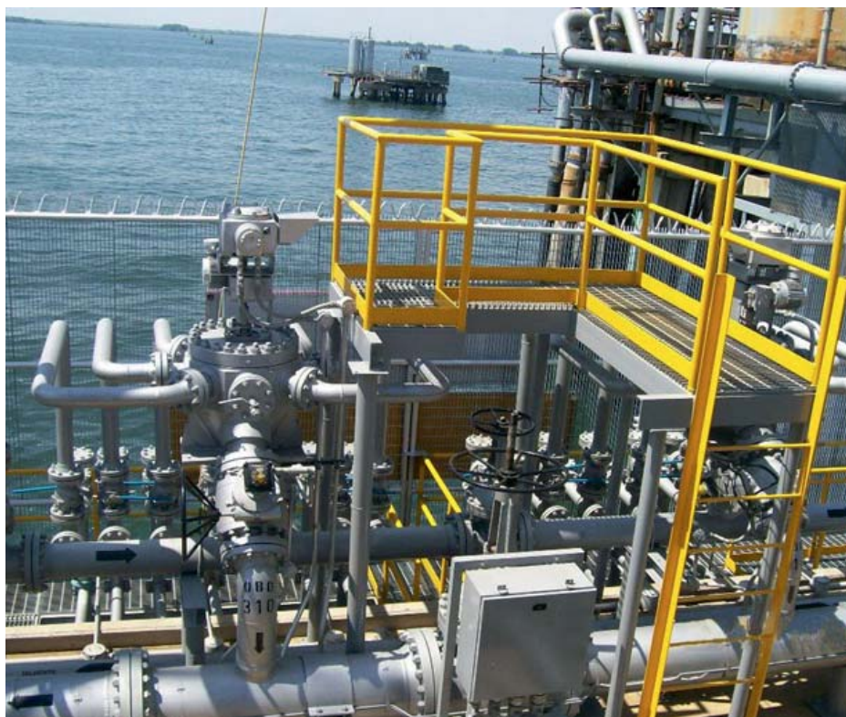
Fig. 4: Multiport Selector Valve in fixed platform
