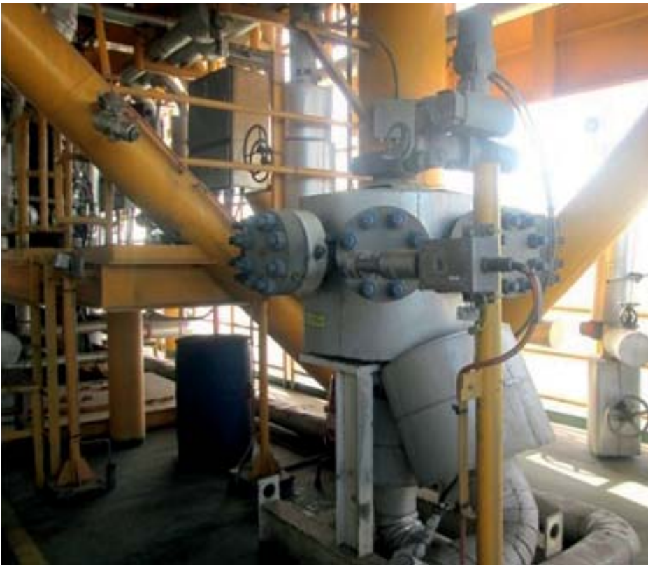
Fig. 8: Multiport Selector Valve on Offshore Platform
